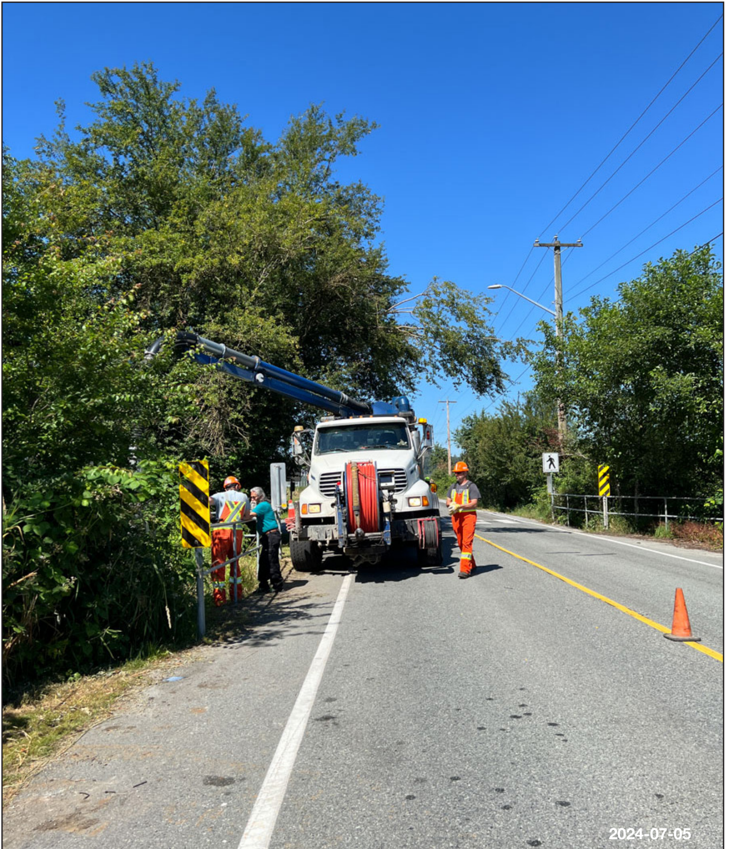
A pump truck was set up above the culvert on Bateman Road.
